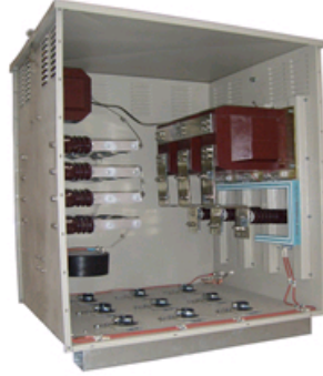
Generator Notr Cubicle 6,3 kV 2000 A with Neutral Grounding Resistor
