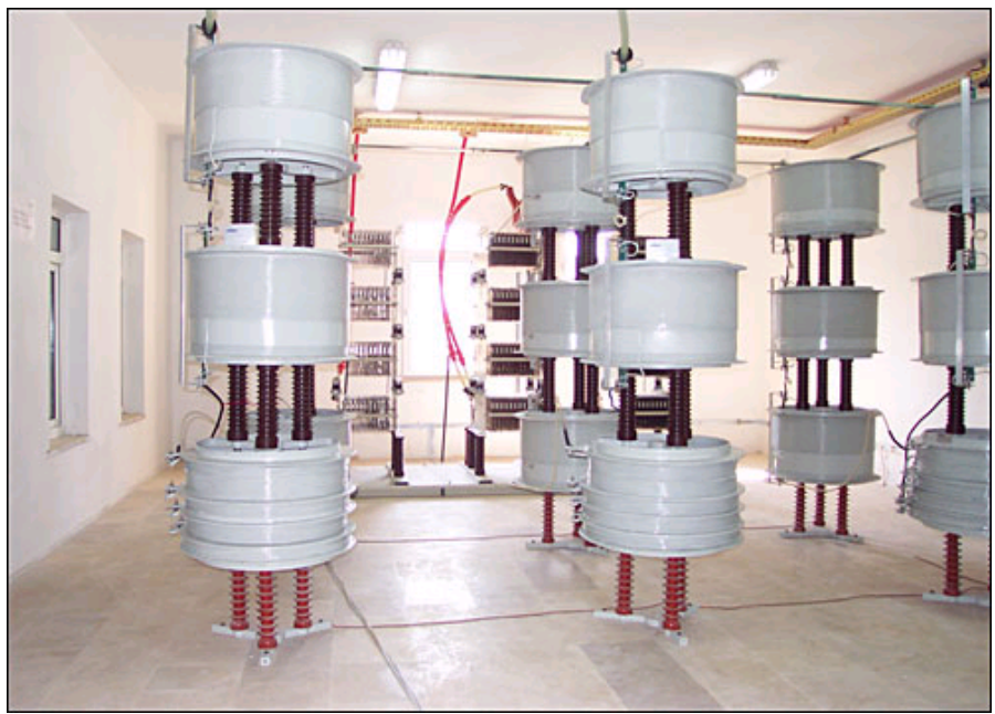
Current Limiting Reactors and Resistors in a Short Circuit Test Laboratory
